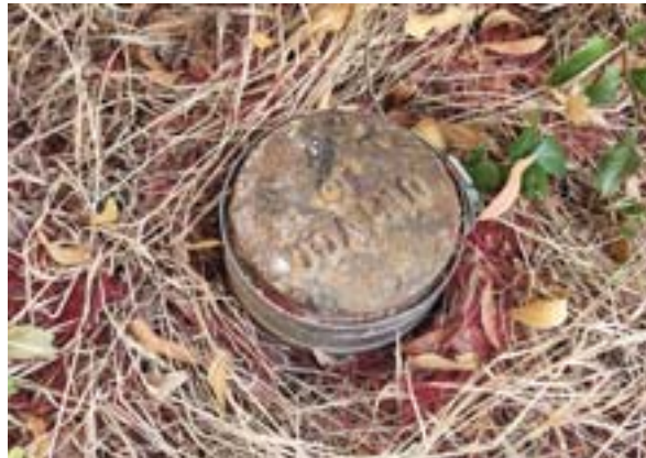
Main Sewer Clean Out
